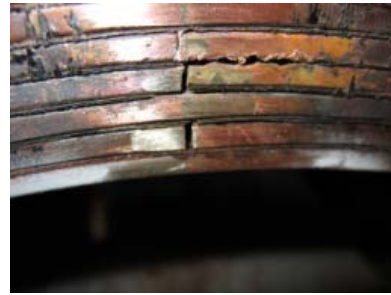
Cracked Winding-Turn Brazes As Found
